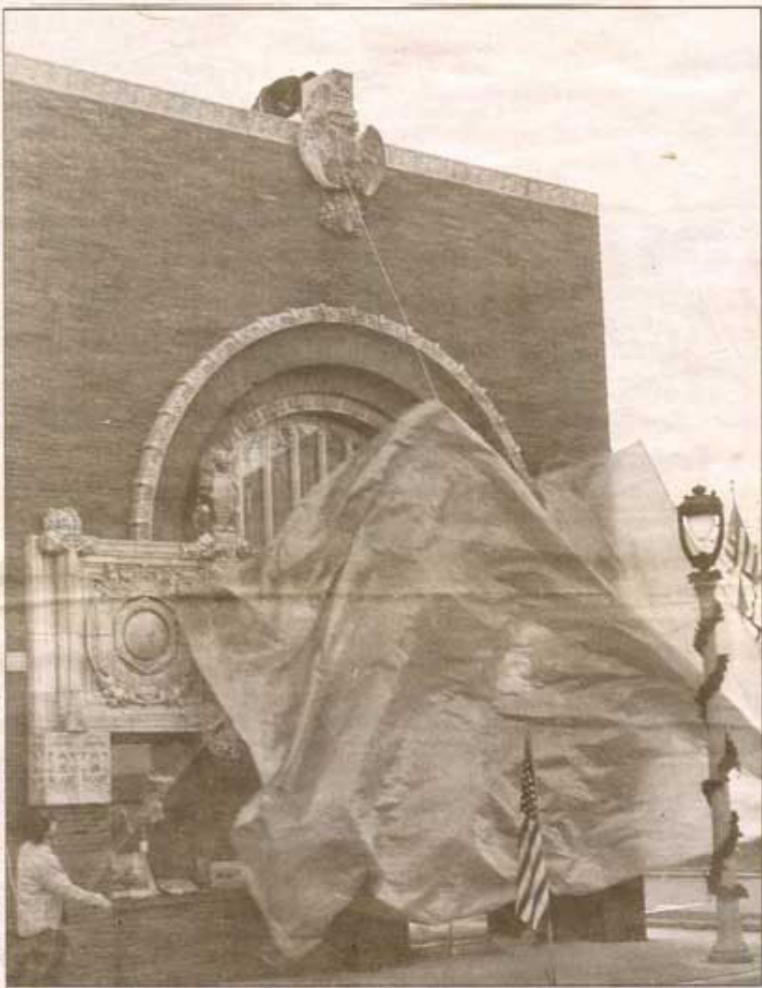
The unveiling of the Farmers and Merchants Union Bank facade on Wednesday at 3 p.m. The bank front has been under construction for over a year
